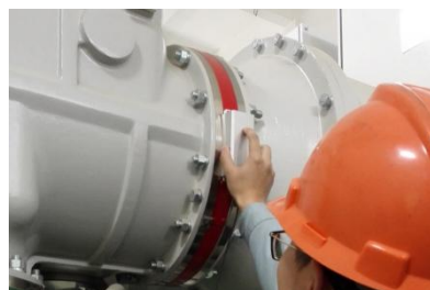
GIS field partial discharge test
